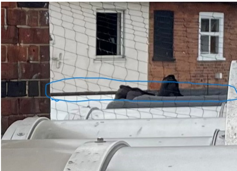
I speculate that course of black bricks to the left of the image that is in line with the end of the blue line highlight the parapet upstand is the same course of brick in the photos between, on the Town Hall that runs two courses of brick above the coping to the top of the Courtyard walling.
