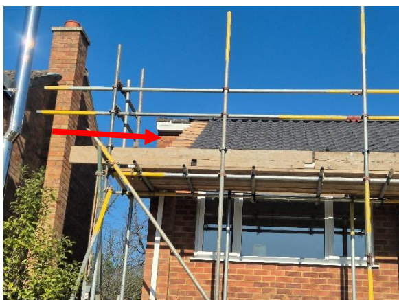
Photograph 13: Gaps on the western elevation of B1 due to incomplete re-roofing, leading into the loft void.
