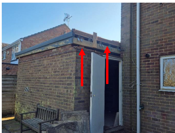
Photograph 17: Gaps within the external walls of the garage of B1, as a result of the partial garage conversion.
