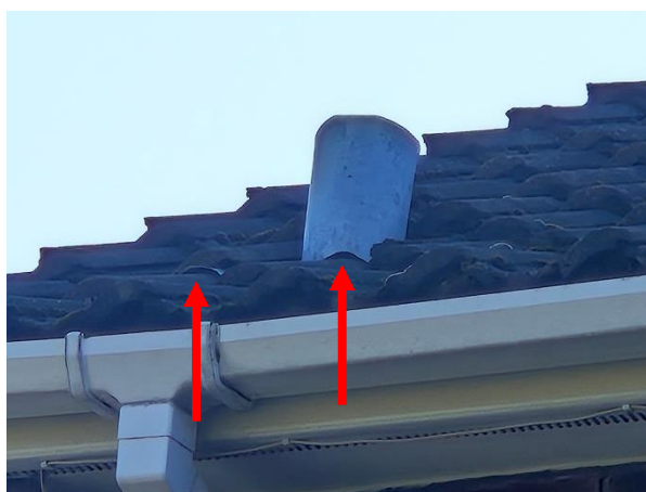
Photograph 15: Gaps beneath flashing on the northern elevation of B1.
