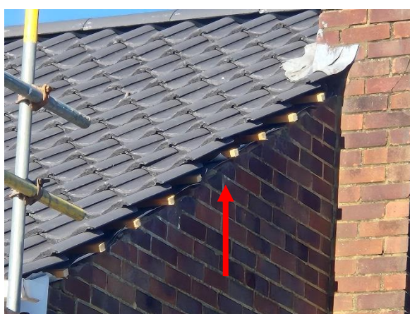
Photograph 14: Gaps on the eastern elevation of B1 due to incomplete re-roofing, leading into the loft void.
