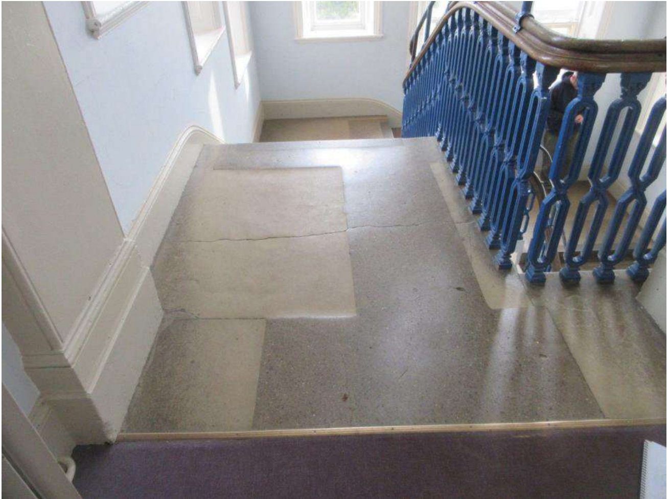
Figure 5. The crack across the full width of the first floor landing, viewed from above. The worn granolithic screed finish is visible to the top surface.
