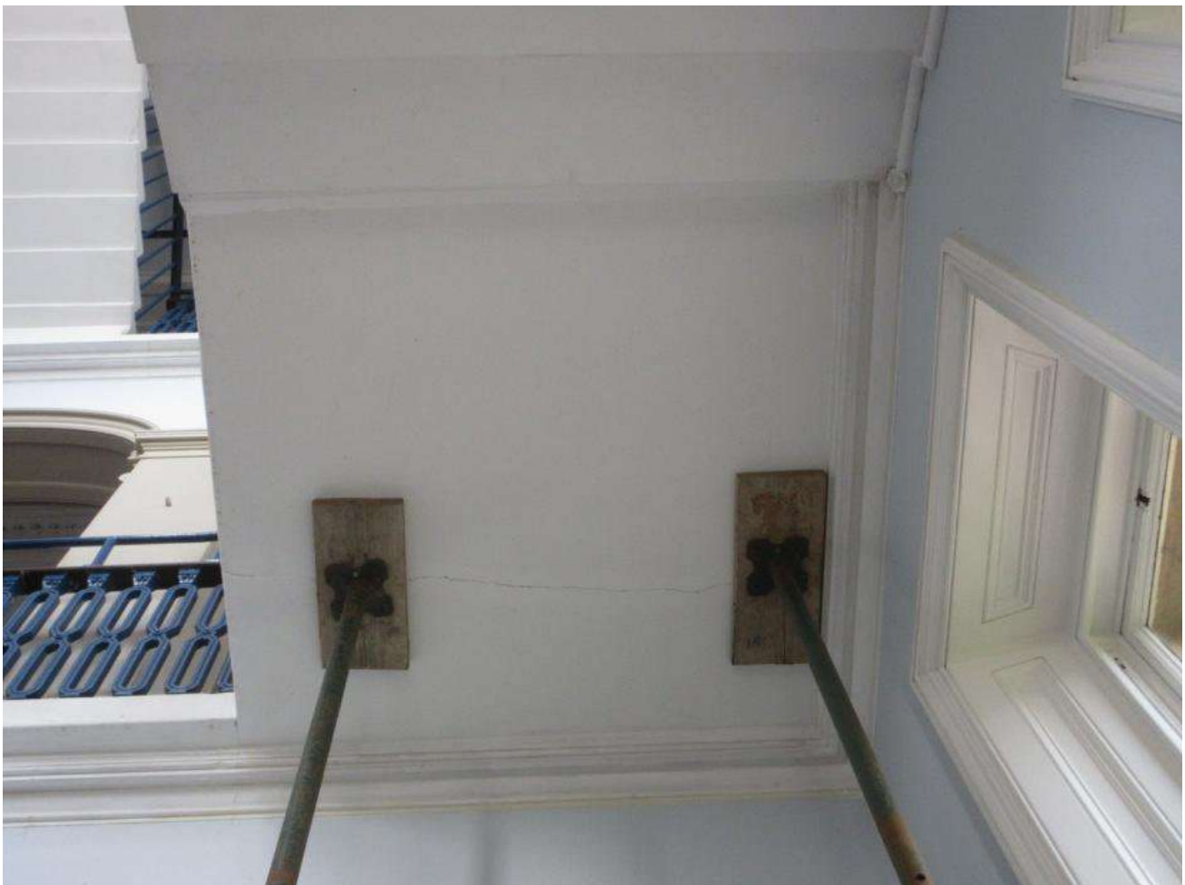
Figure 4. The crack to the first floor landing viewed from below, with Acrow props relocated to provide access.
