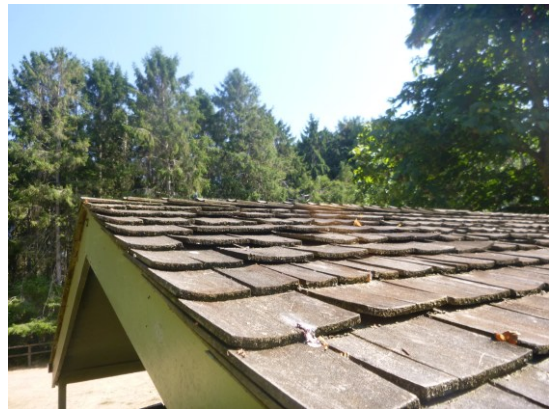
8. Timber shingle roof on summerhouse with some slightly warped shingles (B2).
