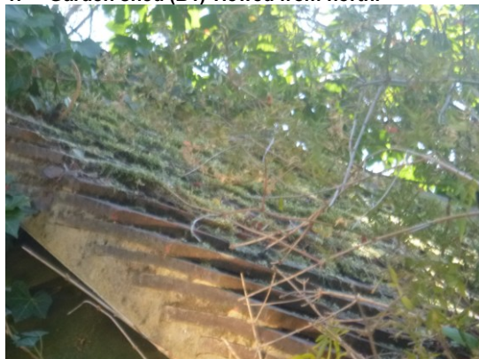
3. Inspected gaps under uneven verge tiles at western gable end (B1).
