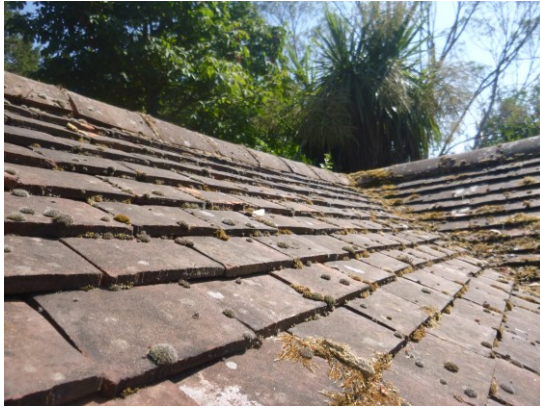
5. Superficial gaps in ridge mortar (B1).
