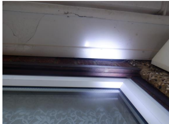
Photograph 9. Gap between uPVC soffit & brickwork (front elevation).
