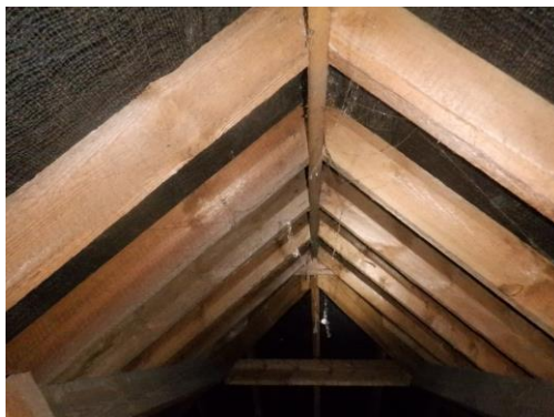
Photograph 10. Ridge cobwebbed throughout the void.
