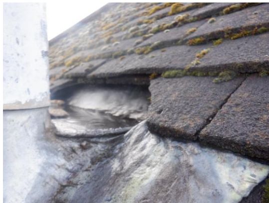
Photograph 7. Superficial crevice beneath cut roof tile (northwest elevation).
