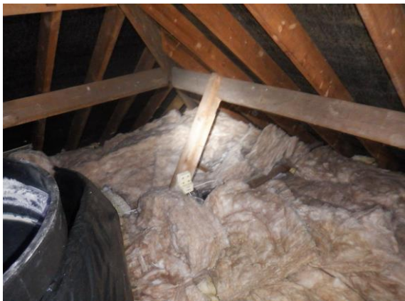
Photograph 13. Eaves blocked by fibreglass insulation.
