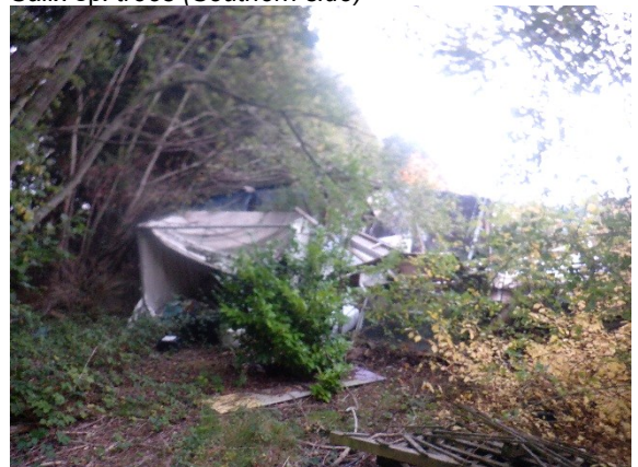
Photograph 4. Dilapidated shed at the south-western corner of the site.
