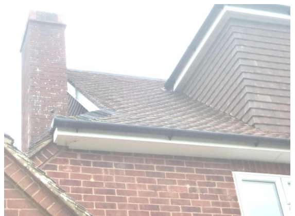
Photograph 7. Gaps behind hanging tiles along the corners of the rear dormer window (rear elevation).
