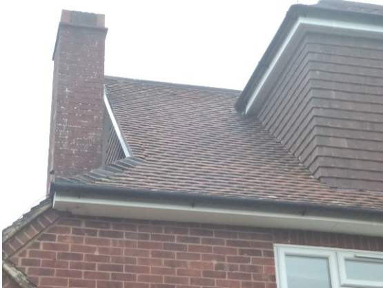
Photograph 2. Gaps under curved roof tiles (rear elevation).
