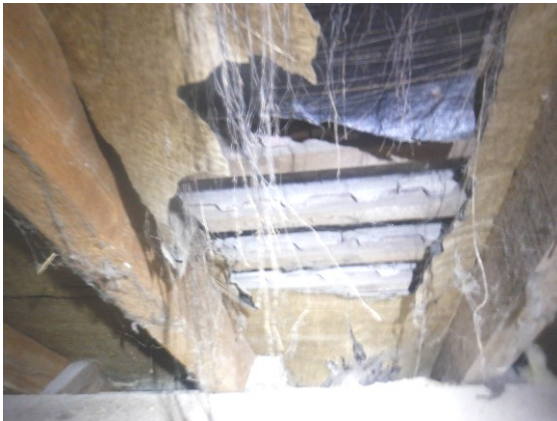
Photograph 9. Torn paper-back felt (Eaves Space 1).
