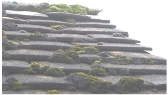
Photograph 3. Lifted clay roof tile at verge of existing extension (north elevation).
