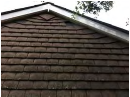
Photo 66 Building B2 – missing tile
