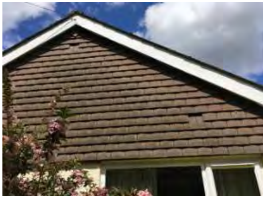
Photo 64 Building B1 – missing tiles
