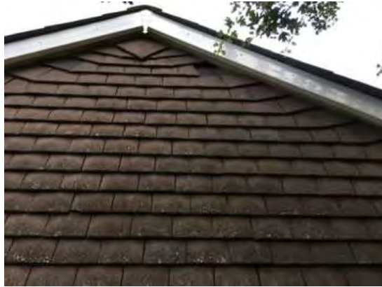
Photo 95 Bird nest behind missing tile on B2
