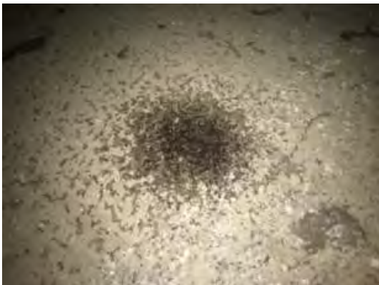
Photo 72 Building B3 – clustered bat droppings
