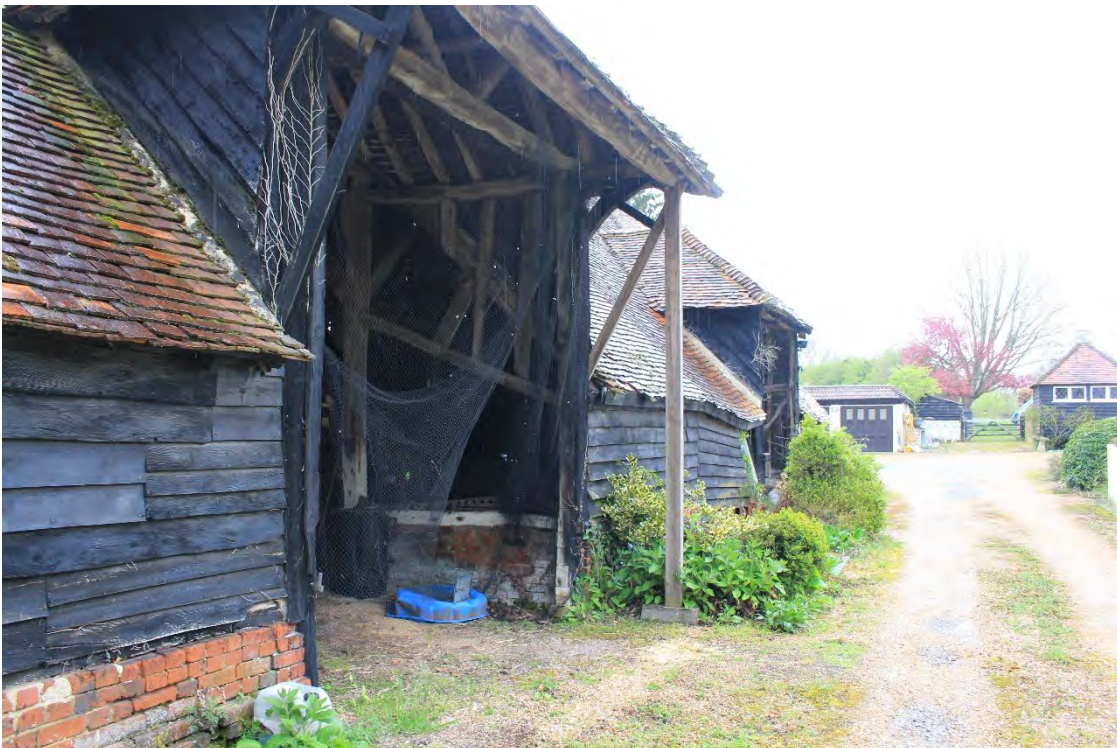
Image EDP A1.12: North-east facing view from the driveway to Pearce's Farm. Image to illustrate the condition and modern brick repairs (bottom left) visible along the exterior of the listed barn ( 1118118 ) at Pearce's Farm.
