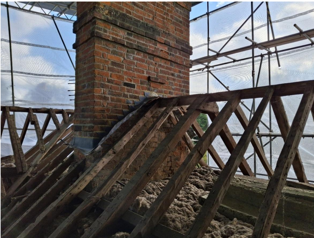
Figure 3: Exposed roof beams and remaining chimney
