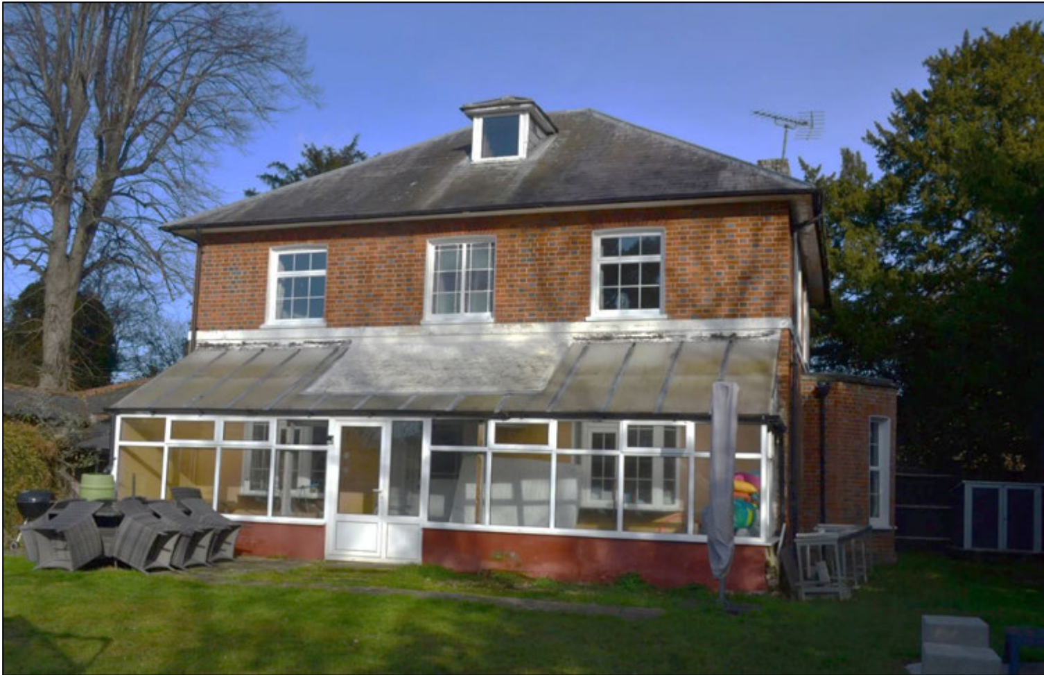
Figure 18 - The conservatory along the south elevation has been in situ in one form or another since the late 19 th /early 20 th century. The roof is currently in poor condition having been very heavily repaired with flashband and sealant. Beneath this in the central part of the roof there are evidence of tiles, which may contain asbestos.
