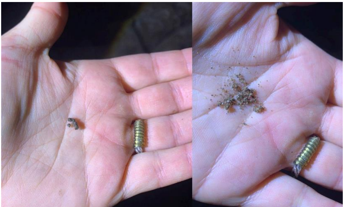
Image 11 – Evidence from bats in the form of 100+ bat droppings across the floor areas to the main roof void spaces of the dwelling
