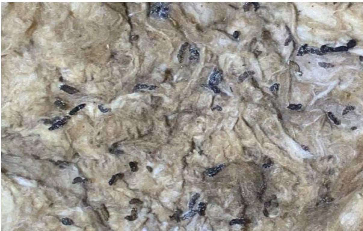
Image 10 – Evidence from bats in the form of 100+ bat droppings across the floor areas to the main roof void spaces of the dwelling
