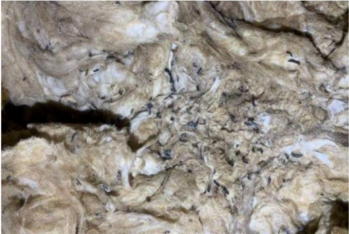
Image 11 – Evidence from bats in the form of 100+ bat droppings across the floor areas to the main roof void spaces of the dwelling
