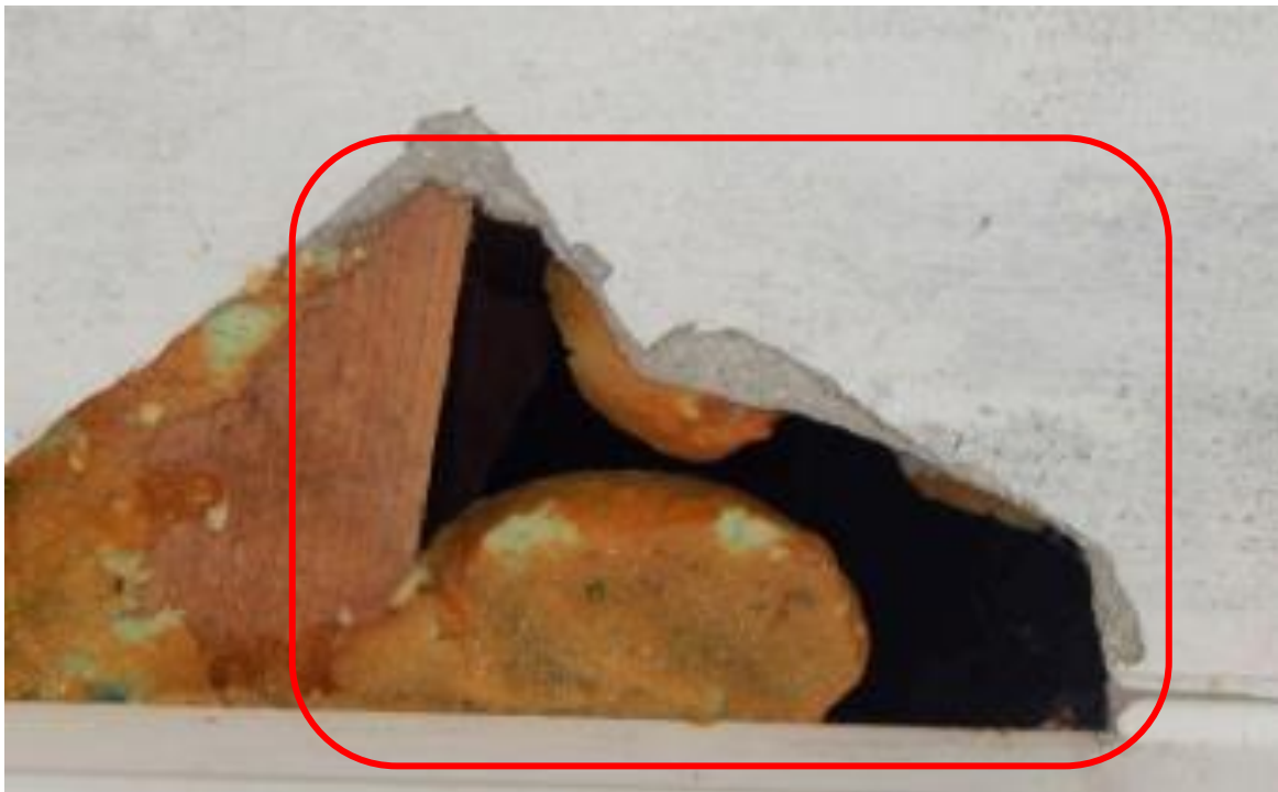
Image 6 – Gaps to the eaves coverings of the front and rear areas of the property of adequate proportions to offer access opportunities for bats and nesting birds within
