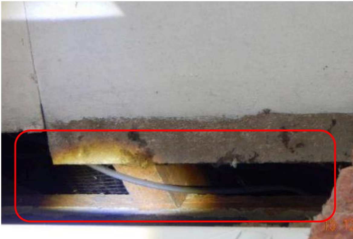
Image 7 – Further gaps to the eaves coverings offering adequate access opportunities into the main roof void spaces of the main dwelling
