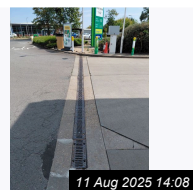
Ref #33.1 - Aco channel drain to site entrance from A4 London Road
