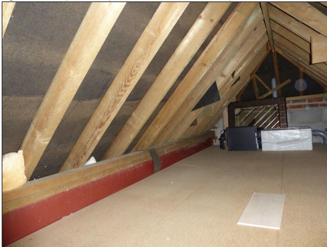
Figure 14. Example of loft space. 23b Pine Drive, Finchampstead, 02.07.24
