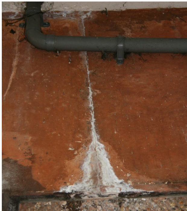
Example of Defect Type H1
