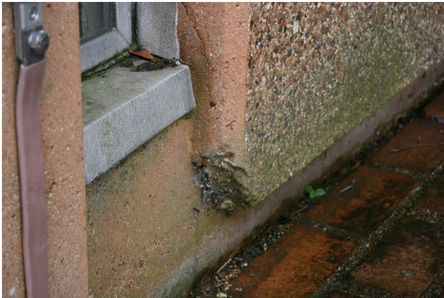
Example of Defect Type B3
