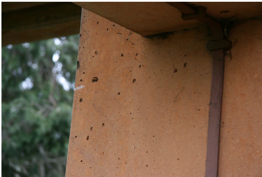
Example of Defect Type B4
