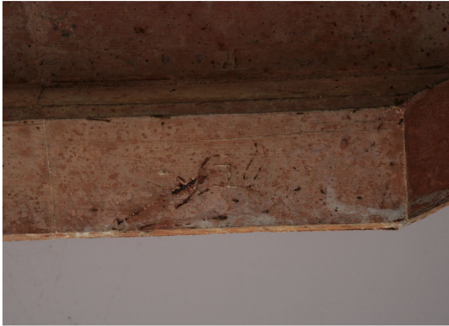
Example of Defect Type B6
