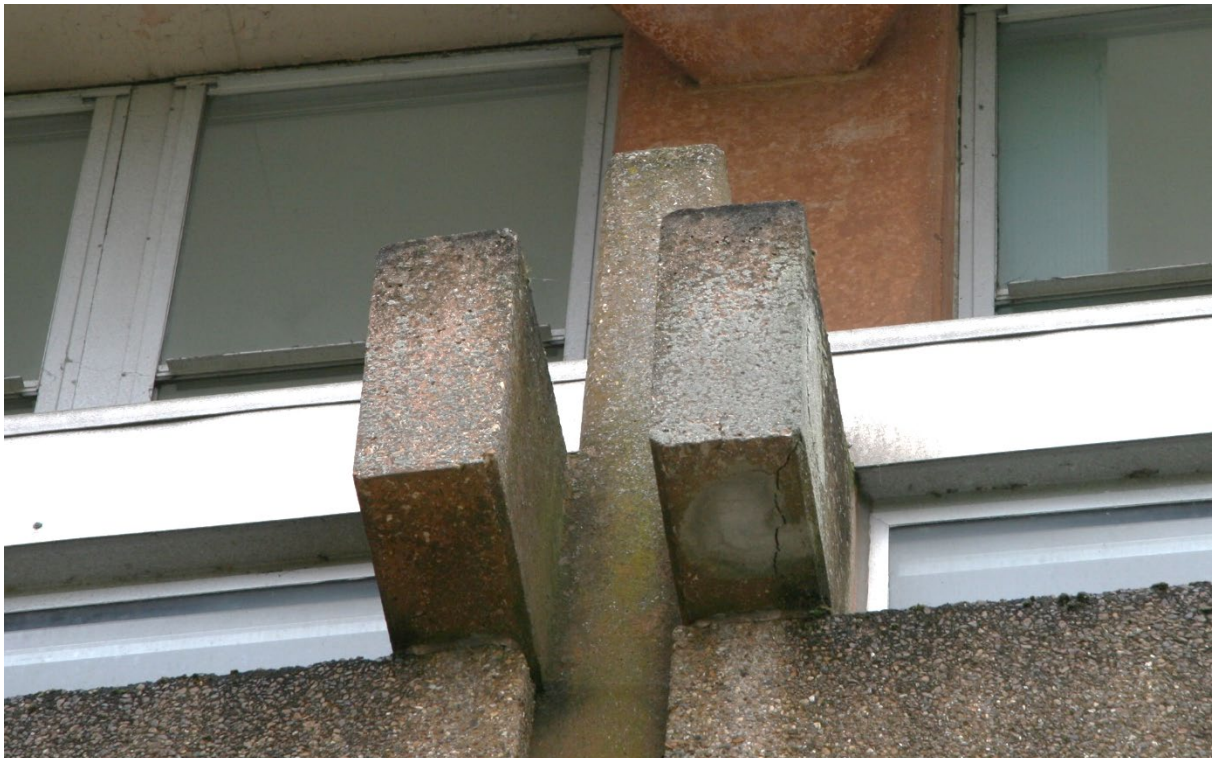
Example of Defect Type A2
