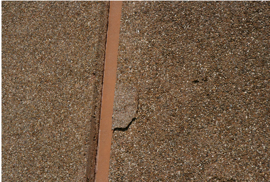
Example of Defect Type B2
