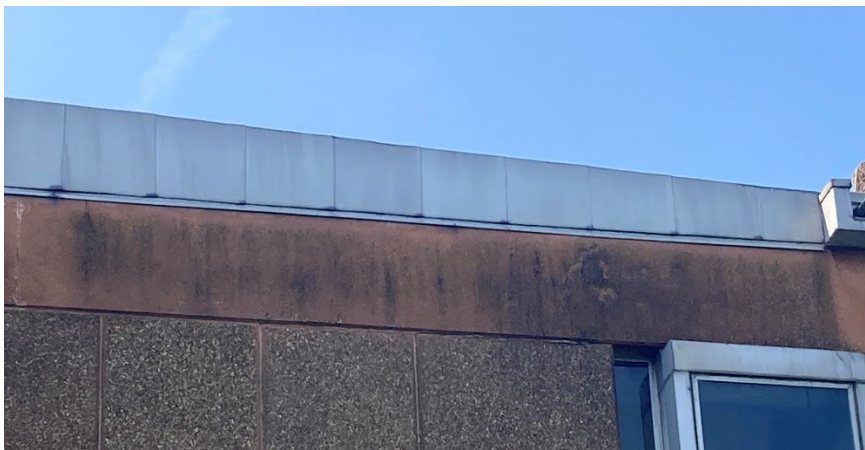
Example of Defect Type S1
