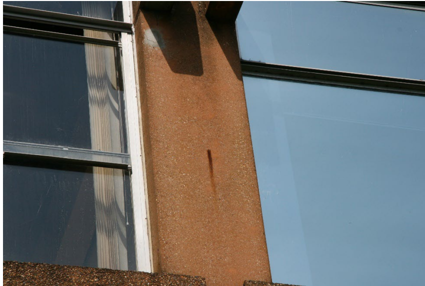
Example of Defect S2
