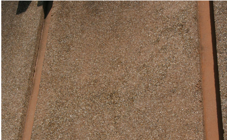
Example of Defect Type B7
