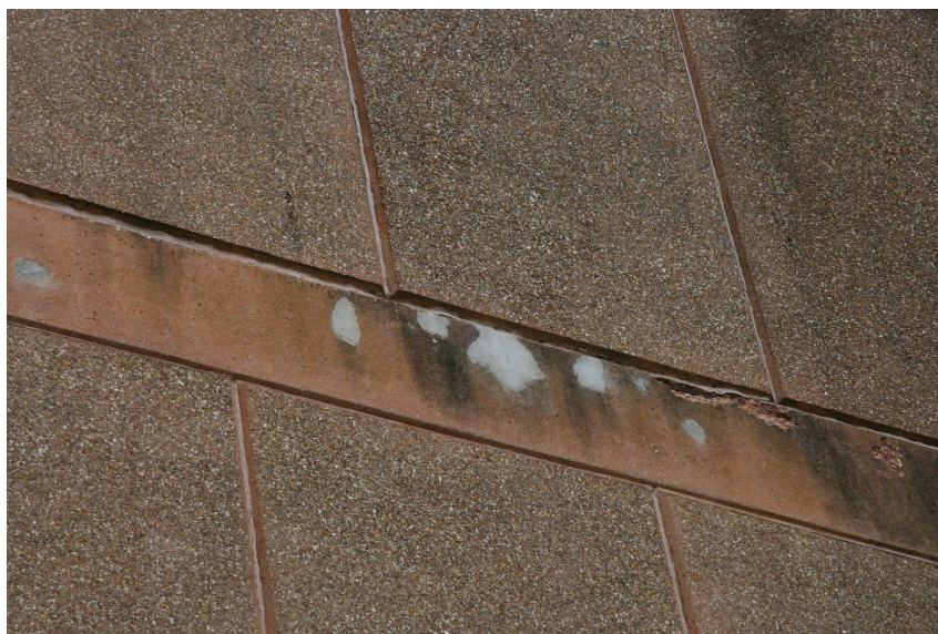
Example of Defect Type C1
