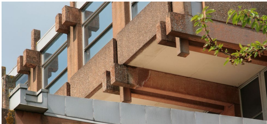
Example of Defect Type H2
