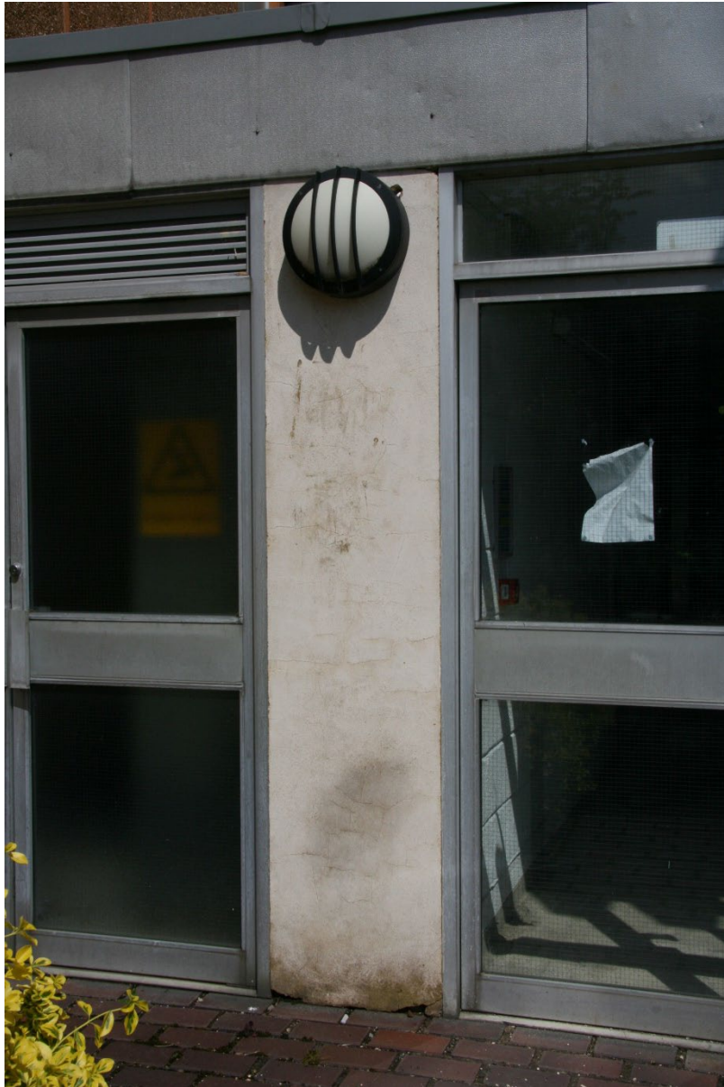
Example of Defect Type J1
