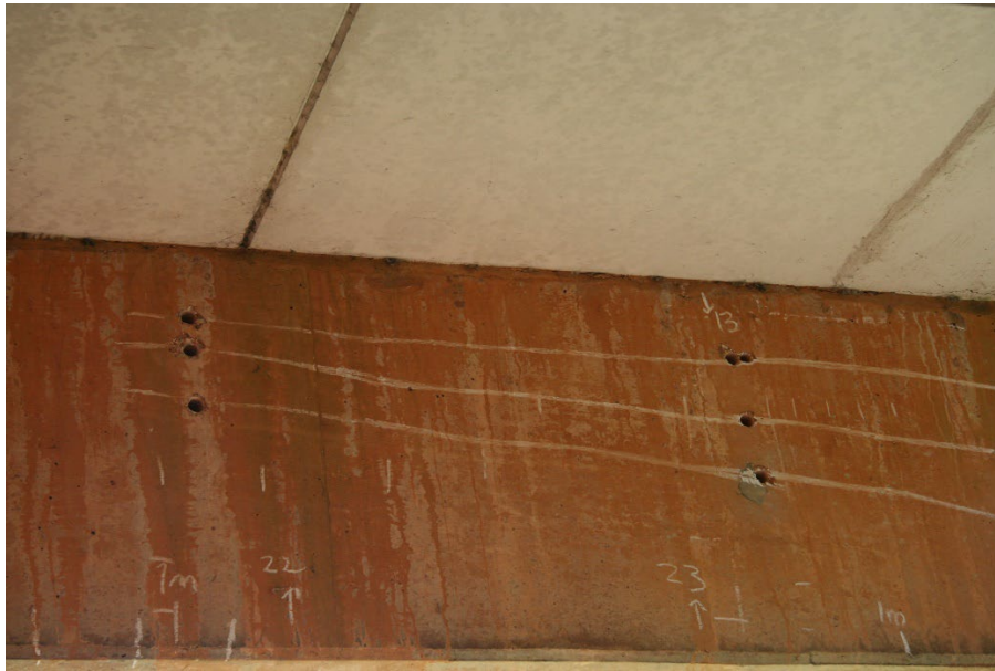
Example of Defect Type D3
