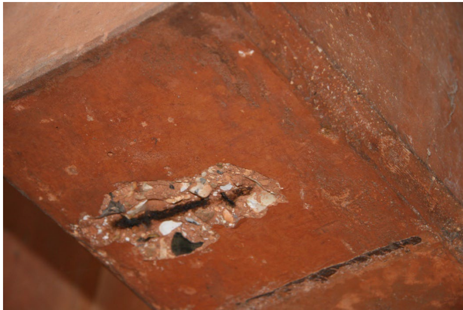
Example of Defect Type B1
