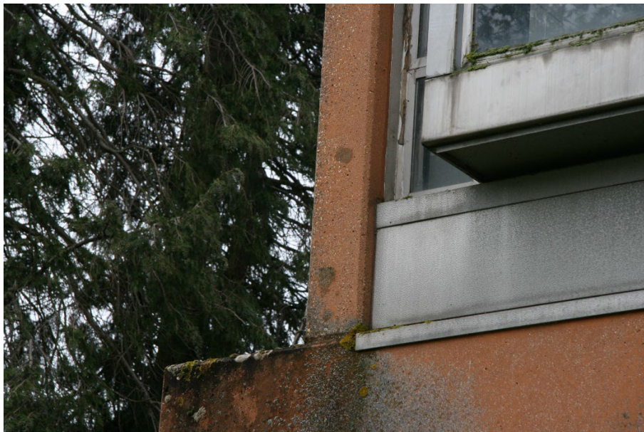
Example of Defect Type C2
