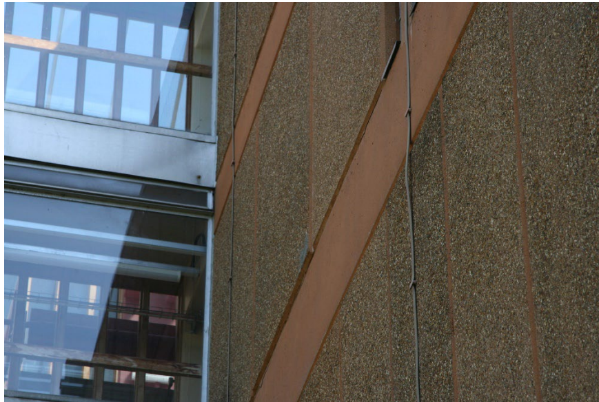
Example of Defect Type E1
