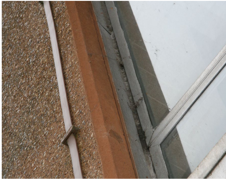
Example of Defect Type K1
