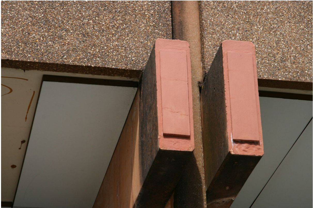
Example of Defect Type A1
