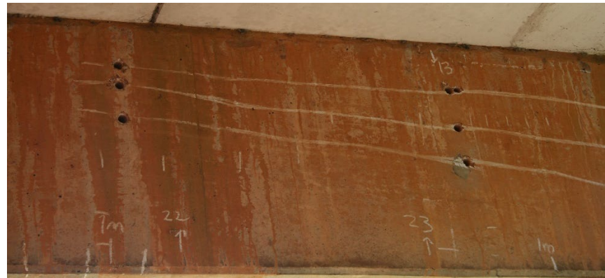
Example of Defect Type D3
