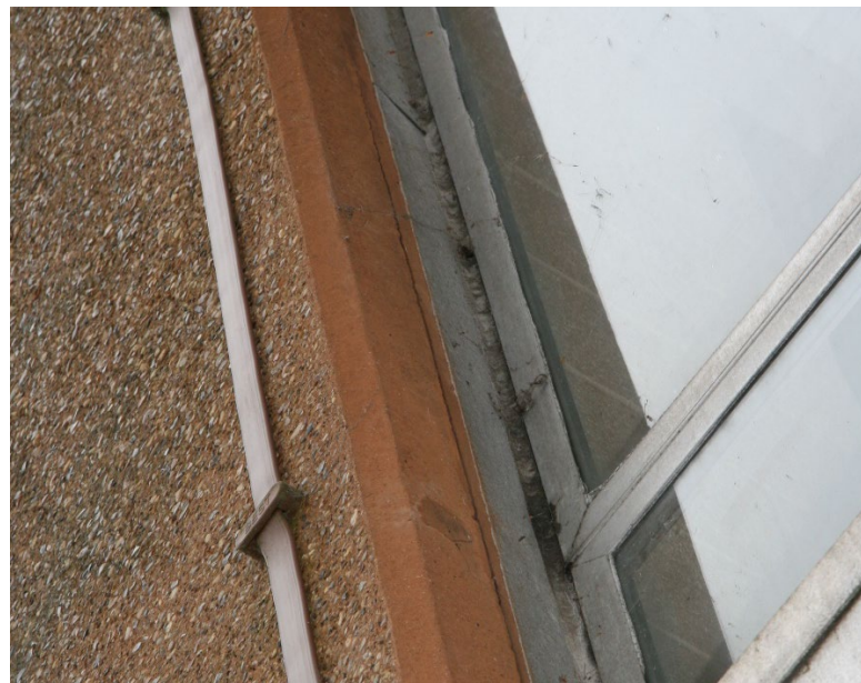
Example of Defect Type K1
