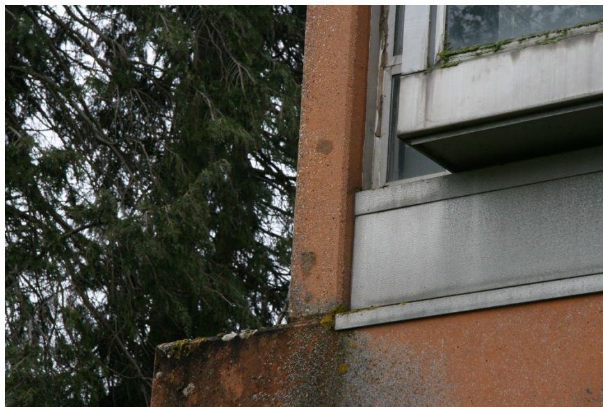
Example of Defect Type C2
