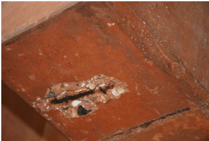
Example of Defect Type B1
