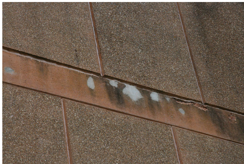
Example of Defect Type C1
