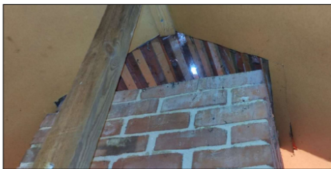
Figure 9 – Roof void above extension to the rear, with no insulation fixed on top of bitumen felt
