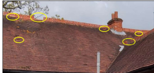
Figure 15- showing missing tiles, gaps at ridge and lack of flashing in the valley
