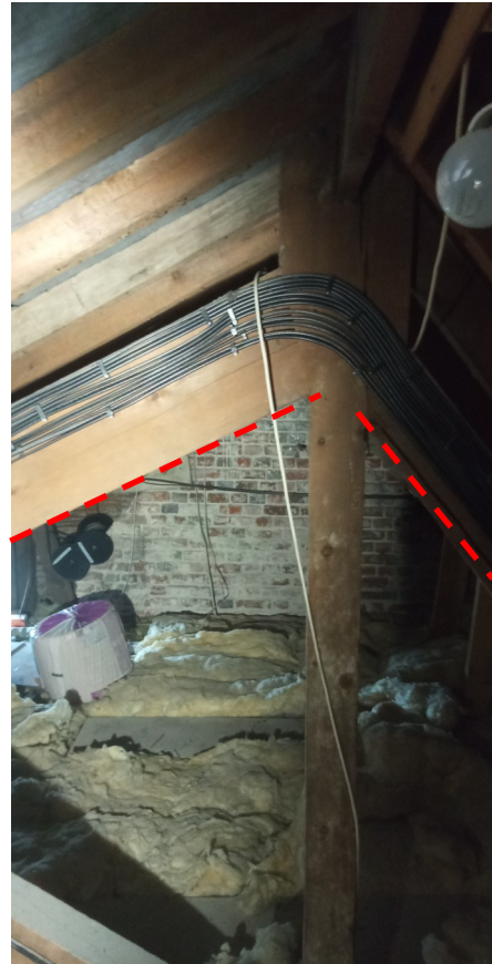
Photo B: view showing the different front and rear roof pitches
