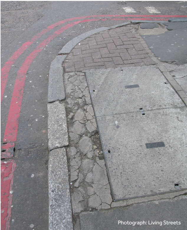
Poor quality pavement
