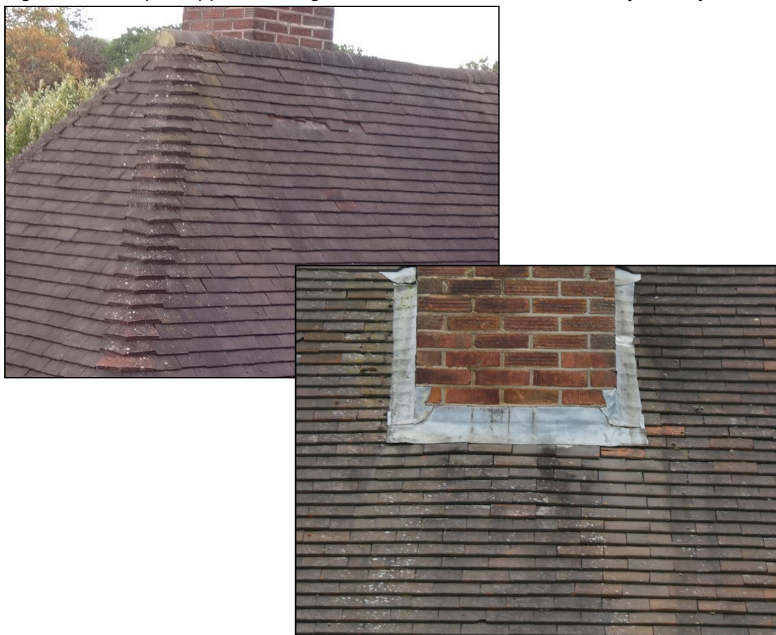
Figure 4. Example slipped/missing/raised roof tiles. 3 Buckhurst Way, Earley. 26.08.25
