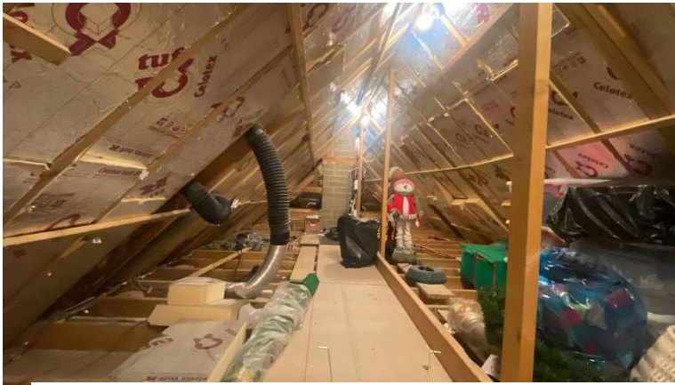
Photograph 10: Loft Void penetrations of CHH
