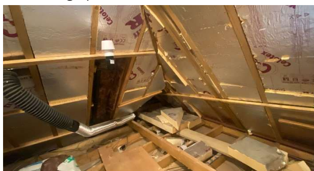
Photograph 9: Loft Void penetrations of CHH
