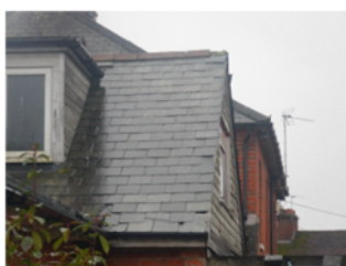
3. Multiple gaps from slipped slate tiles.
