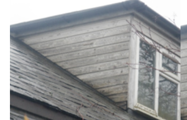
6. Gap behind timber cladding of dormer.
