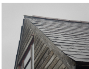
4. Missing edge ridge tile on western elevation.
