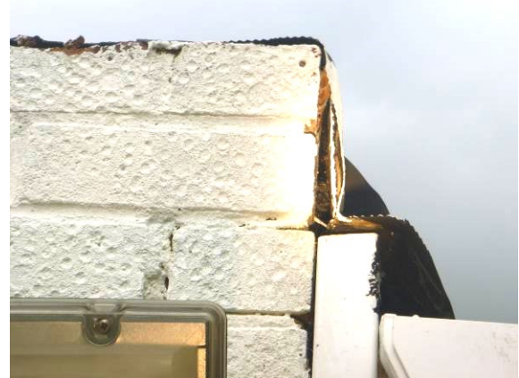
Photograph 8. Gap behind roofing felt at corner of extension (rear elevation).
