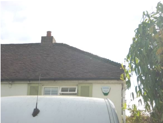
Photograph 3. Uneven clay tiles (front elevation).
