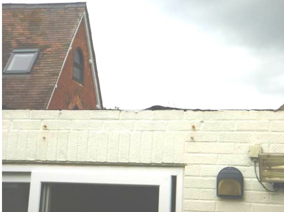
Photograph 7. Lifted roofing felt bituminous on extension (rear elevation).
