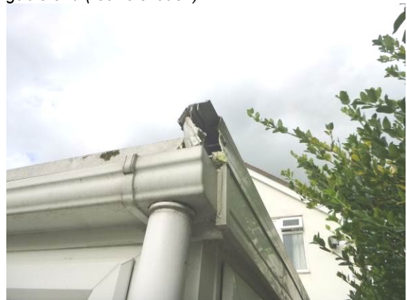
Photograph 6. Hole in conservatory roof (rear elevation).
