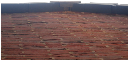
Photograph 7. Gap below the verge cap at the apex (southern elevation).
