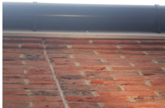
Photograph 6. Barge board tight to brickwork (rear elevation).
