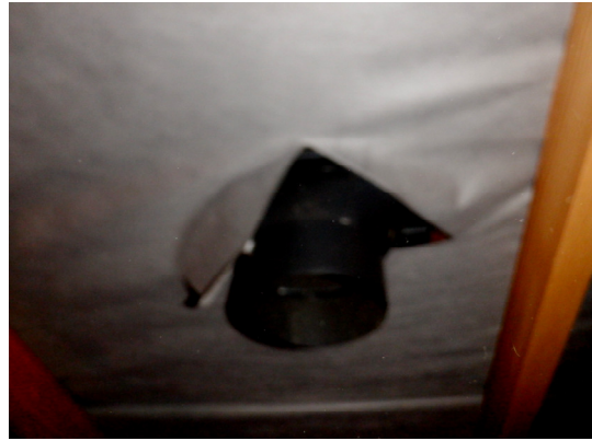
Photograph 9. Tear in breathable roofing membrane around ventilation tile (roof void).
