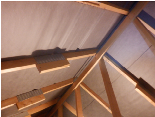
Photograph 10. The cobweb free ridge (roof void).
