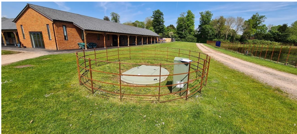
Fig. 1 – Sewage Treatment Plant and power unit, enclosed by estate railings (May 2024)
