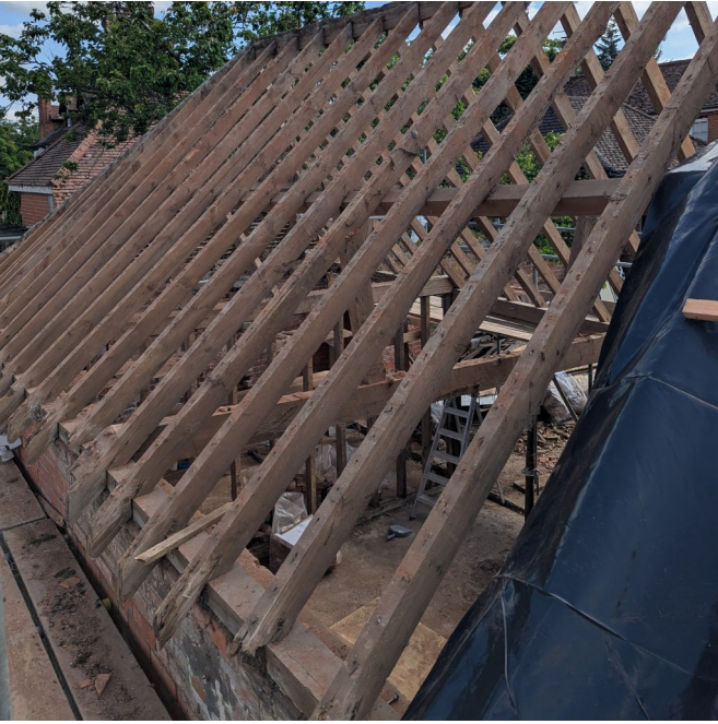
A) Rotten rafter ends
