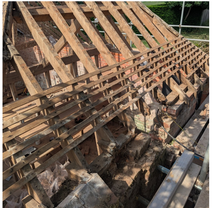
D) Rotten wall plate and rafter ends at wall abutment
