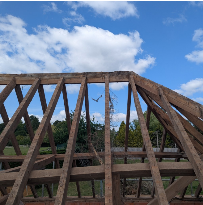
C) Damaged ridge and hip rafters and distortion to purlin
