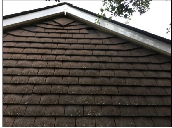
Photo 67 Bird nesting behind slipped tile
