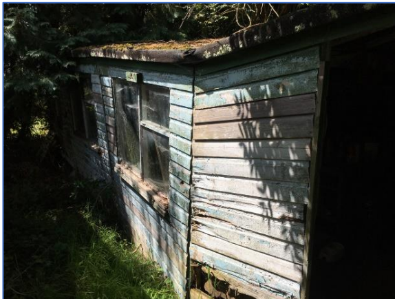
Photo 58 Dilapidated structure (B5)
