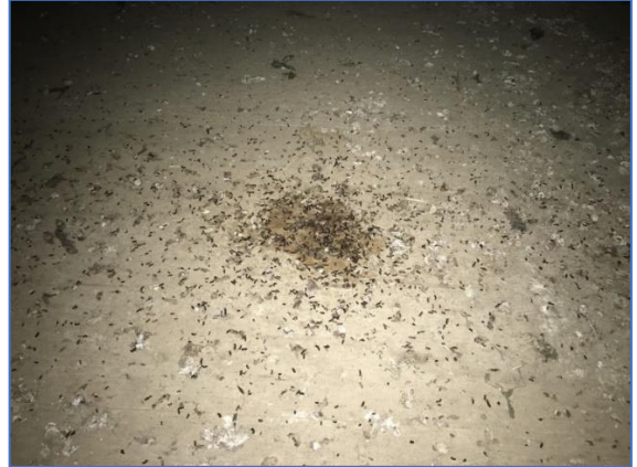
Photo 55 Cluster of bat droppings pile 2 (B3)
