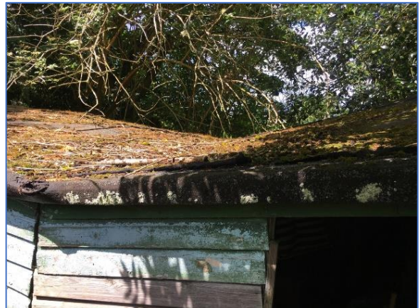
Photo 59 Dilapidated structure (B5)
