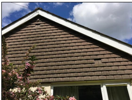
Photo 38 Slipped tiles (B1)
