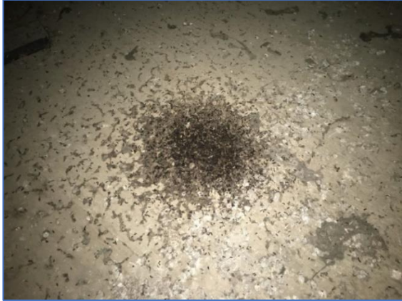
Photo 54 Cluster of bat droppings pile 1 (B3)
