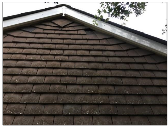
Photo 43 Missing wall tile (B2)
