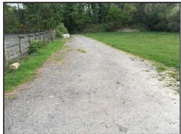
Photo 32 Compressed concrete path A4.
