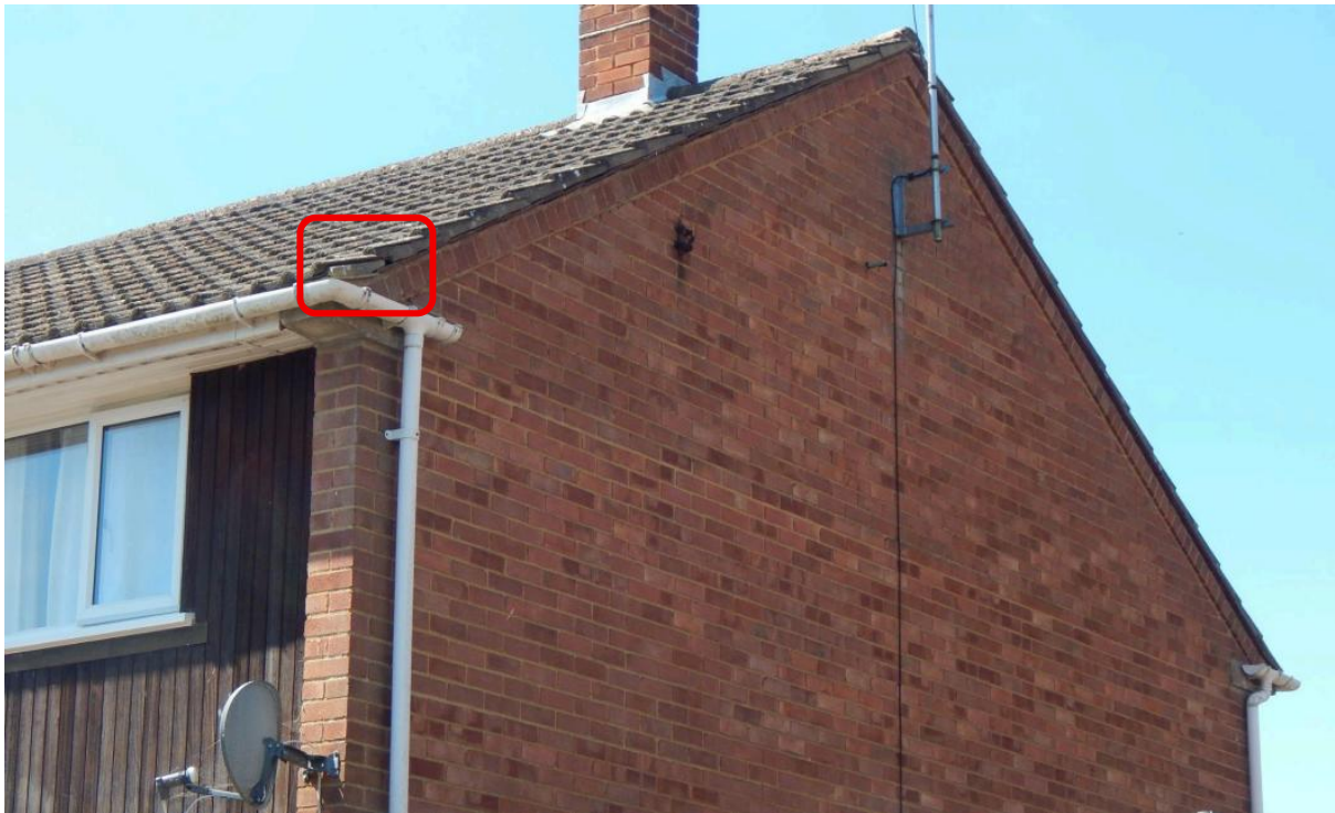
Image 3 – North facing elevation of the property offering a small section of deterioration which looks to provide likely shelter opportunities for bats within
