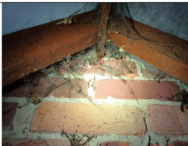
PHOTOGRAPH 8- HIGH LEVEL OF COBWEBBING AT THE GABLE AND RIDGE
