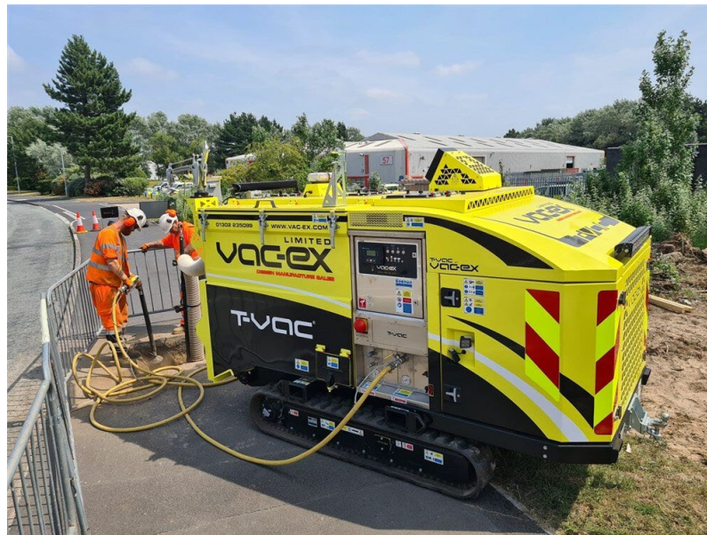
Image of a small Vac Ex and Air Spade combined machine
