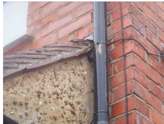
Photograph 9. Crack in render on front porch (eastern elevation)
