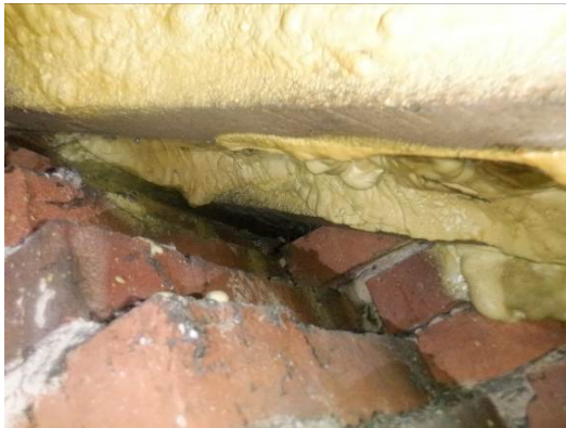
Photograph 11. Small gap between brickwork of party wall and timber rafters (roof void).
