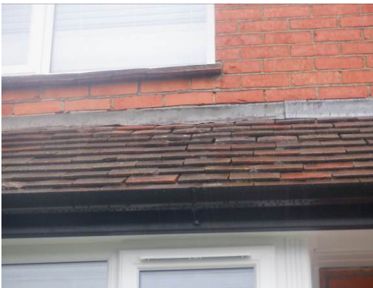
Photograph 8. Uneven overlapping roof tiles and flush lead flashing (northern elevation).
