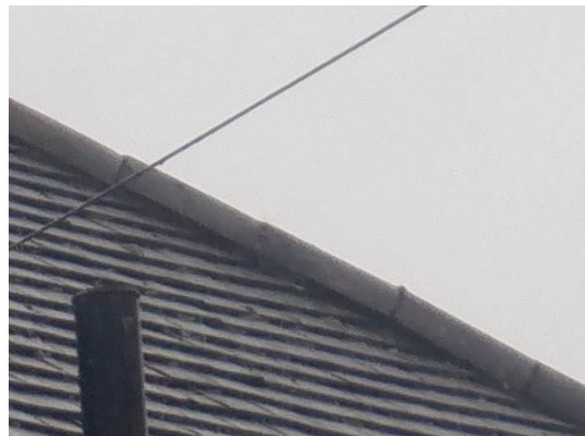
Photograph 4. Small gap in mortar below hip tiles (eastern elevation).
