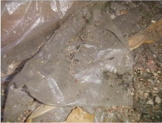
Photograph 14. Small cluster of medium-sized bat droppings (roof void).
