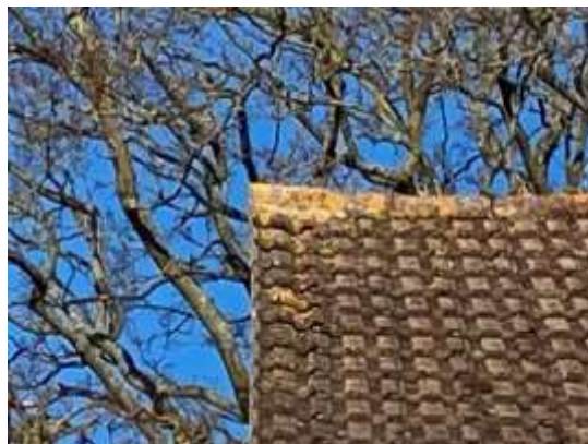
8. Slightly lifted verge tiles on the front elevation.
