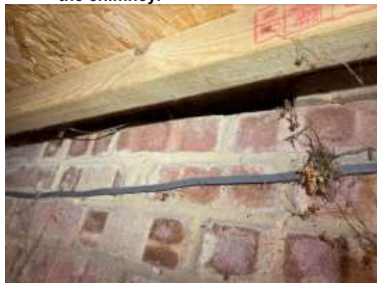
18. Gap between wall and roof on the north eastern side.
