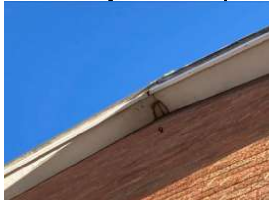
6. The tightly fitted soffits on the side (south west facing) gable end.
