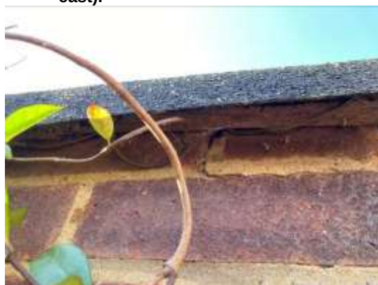
12. Open gap between flat roof and wall on the north eastern side of the garage.
