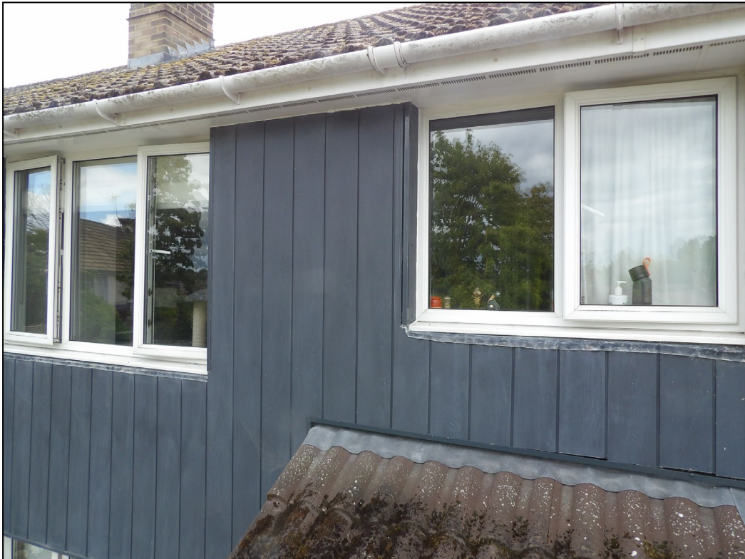
Figure 10. Example sealed wooden cladding. 5 Brook Close, Wokingham. 30.07.25
