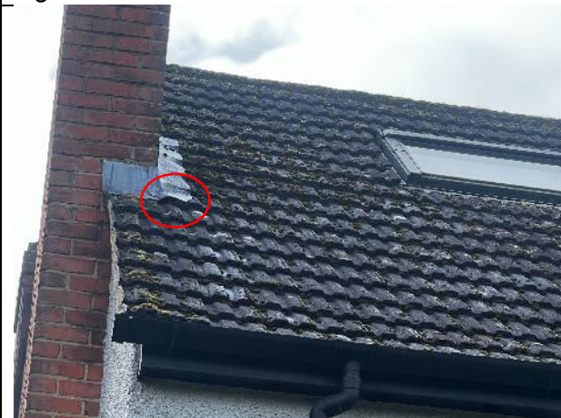
Figure 4: Lifted lead flashing on the east elevation
