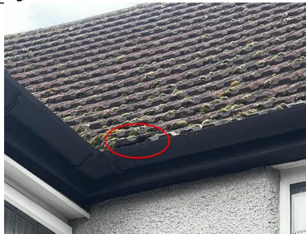
Figure 5: Lifted roof tile on the western elevation
