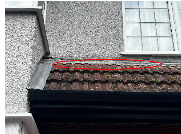
Figure 7: Lifted lead flashing on western entrance porch
