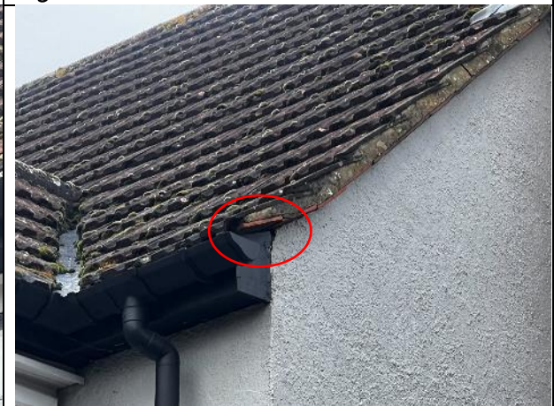
Figure 6: Gap in south-western soffit
