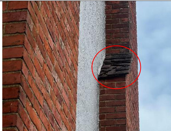
Figure 8: Slipped tiles on southern elevation
