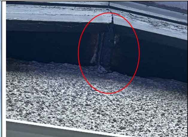
Figure 9: Gap at eaves on western gable apex
