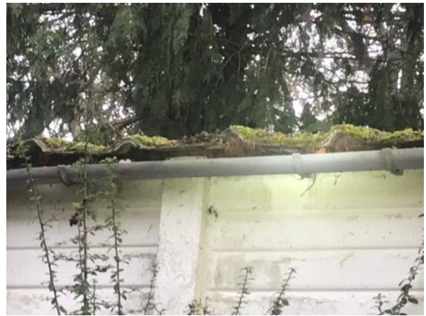
Photo 8: Gap under corrugated roof of building B1
