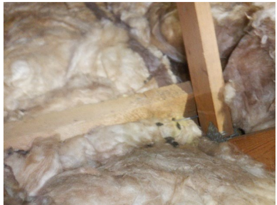
Photograph 11. Rat droppings on fibreglass insulation (roof void).
