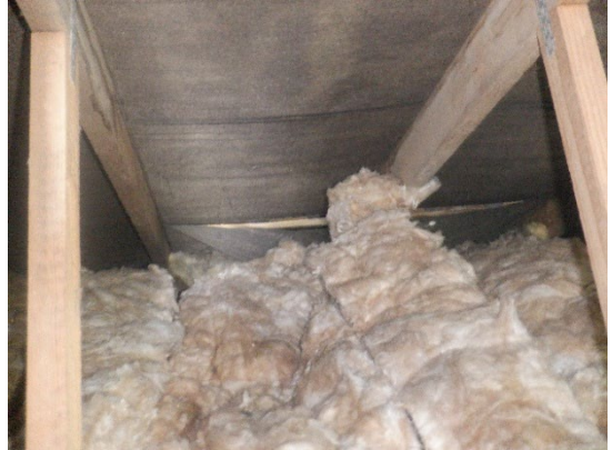
Photograph 9. Loose overlapping section of felt on the rear elevation (roof void).
