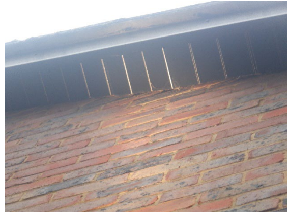
Photograph 6. Gap under uPVC soffit on western gable.
