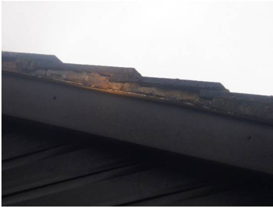
Photograph 5. Crumbling verge mortar above garage (western elevation).
