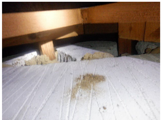
Photograph 13. Blockwork tight to roof felt (roof void).
