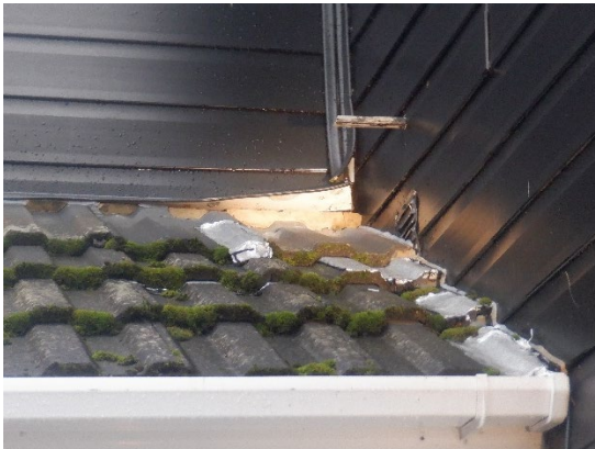
Photograph 7. Lifted uPVC trim above porch roof (front elevation).
