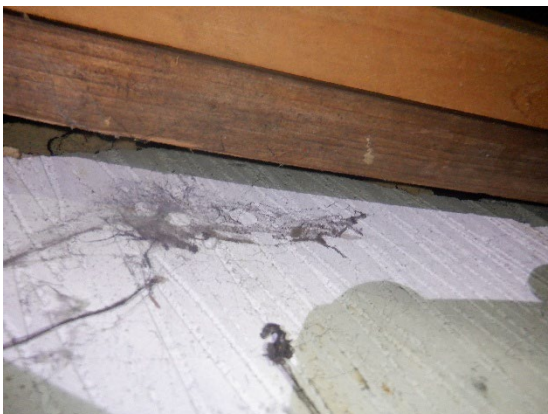
Photograph 12. Cobwebbed blockwork gable (roof void).
