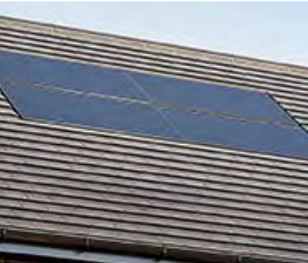
Grey roof tiles with integrated solar panels
