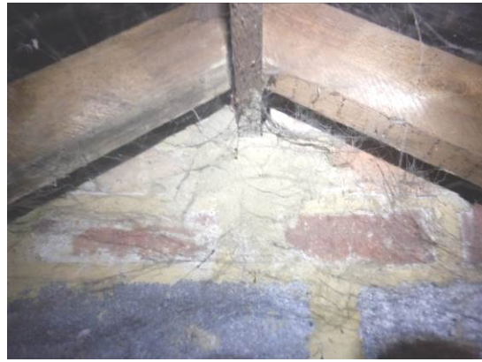
14. The cobwebbed gaps between the end rafter and walls at the gable and party wall and cobwebbed ridge.
