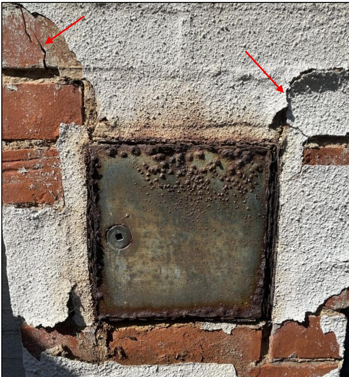
Figure 18. Corrosion and expansion of the metal inspection hatch, with localised cracks developing in the brickwork.
