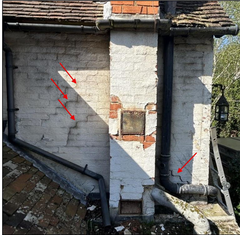
Figure 9. Cracks in the east wall .
