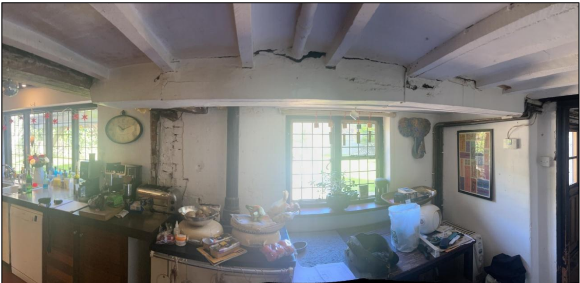
Figure 20. Panoramic view of the south face of the east-west beam with noticeable gaps between the ceiling and the beam, and signs of cracking/fractures within the beam.
