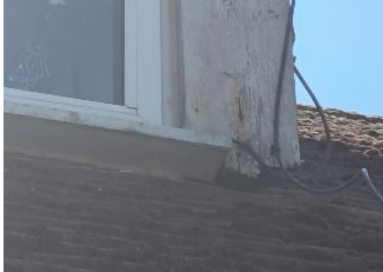
PRF: Rotting wood creating a gap under dormer at the front of the property.
