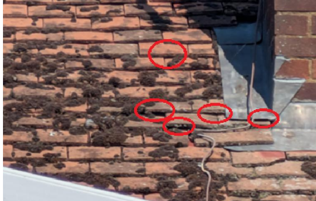
PRF: Raised tiles around chimney and raised lead flashing at the rear of the property.
