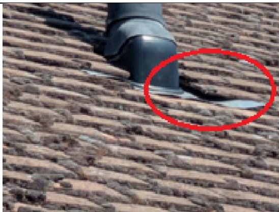
PRF: Raised tiles around the lead flashing at the rear of the property.
