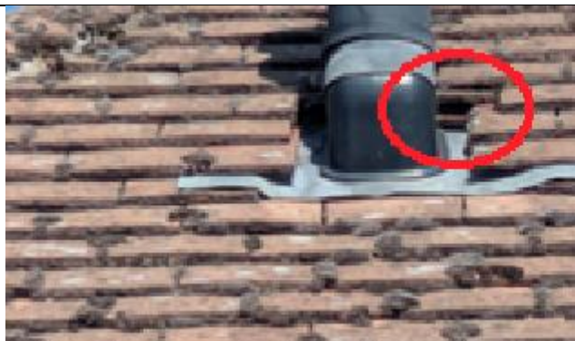
PRF: Raised tiles around the lead flashing at the rear of the property.
