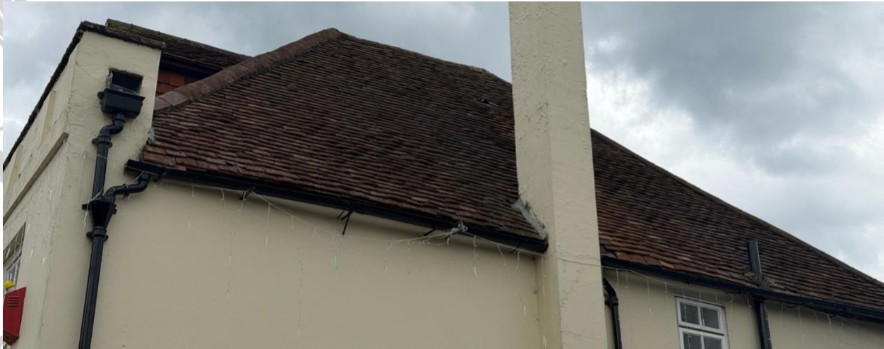
Photograph 1. Clay-tiled roof slope showing multiple raised, uneven and gapped tiles, with potential crevice features beneath tiles and along roof junctions.
