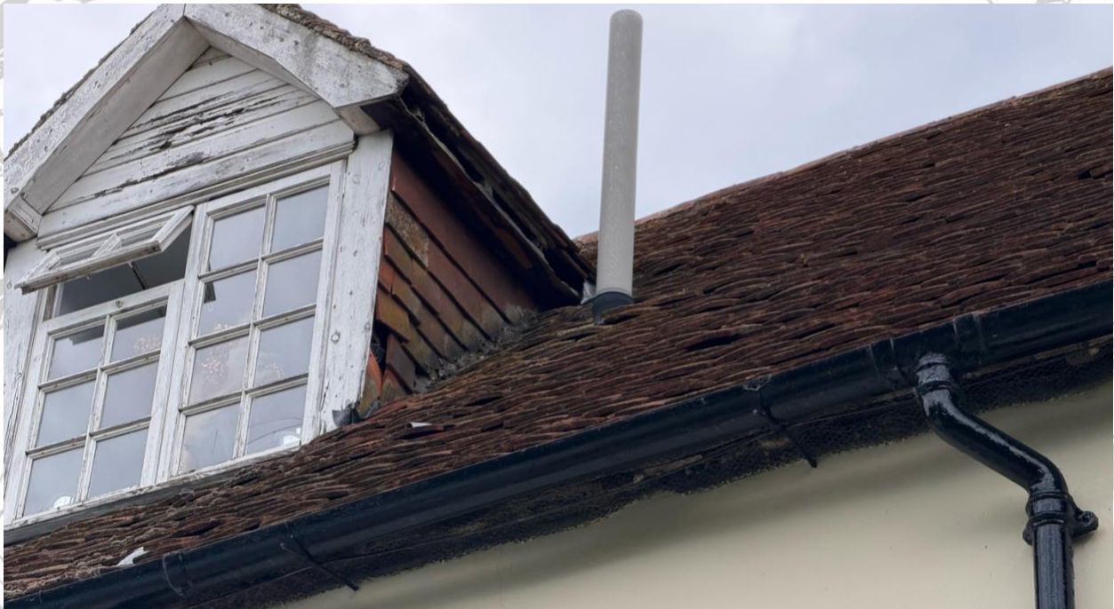
Photograph 4. Dormer and main roof interface showing gaps beneath tiles, weathered timber boarding, and potential roost features around the dormer cheek and roof junction.
