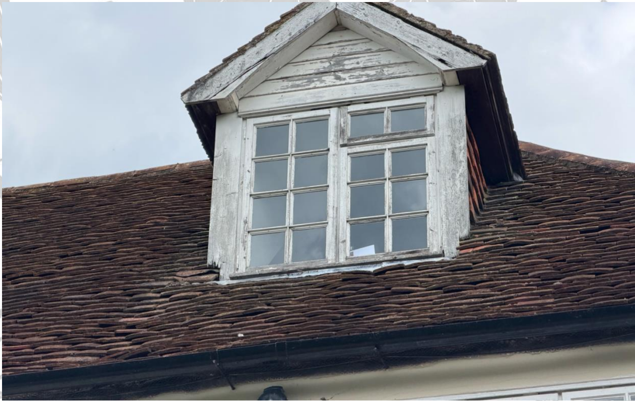
Photograph 5. Dormer window structure showing weathered and deteriorated timber elements, crevices around the window surround, and gaps beneath surrounding roof tiles.
