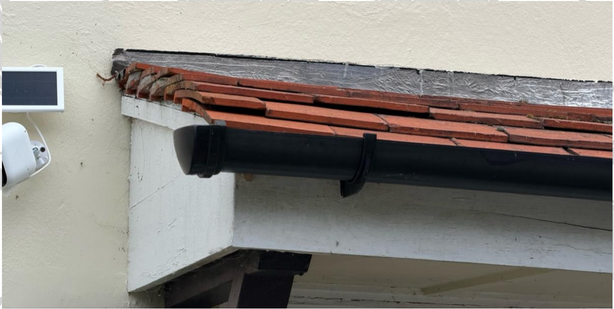
Photograph 7. Lower roof/eaves interface showing raised tiles, gaps beneath tiles and localised access opportunities at the wall and roof junction.
