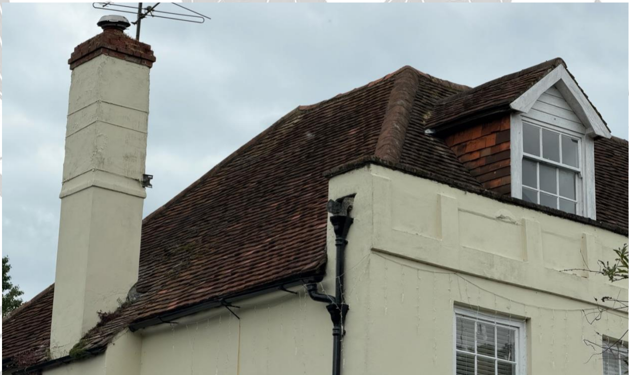
Photograph 9. Chimney and roof slope showing complex roof junctions, ridge and hip tiles, weathered roof covering and potential crevices around roof and chimney interfaces.
