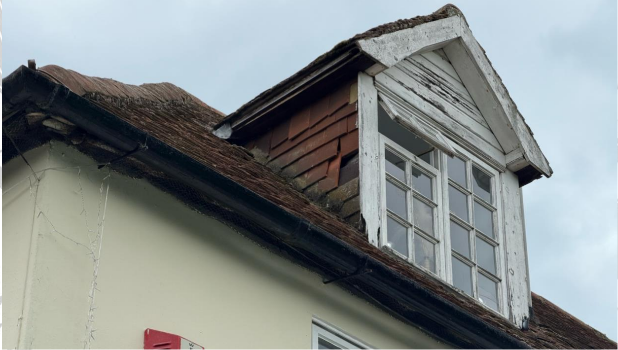
Photograph 3. Dormer window and surrounding roof fabric showing weathered timber, gaps around dormer cheeks, tile gaps and potential crevice features around the dormer interface.
