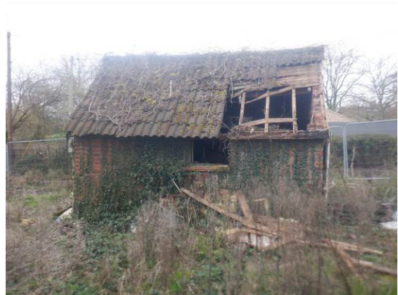
Photograph 10. Dilapidated garage viewed from (east elevation).
