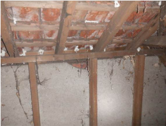
Photograph 13. Asbestos and spray foam at half-hipped gable (roof void).
