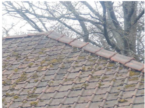
Photograph 4. Crumbling ridge and hip mortar (rear elevation).
