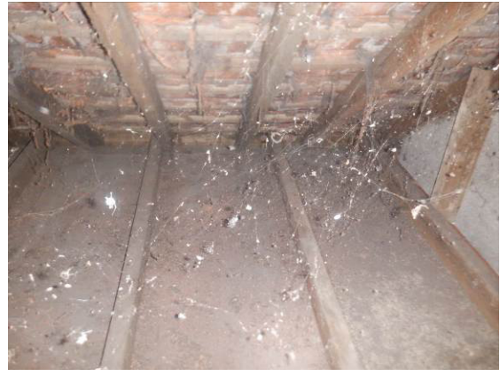
Photograph 14. No floor insulation (roof void).
