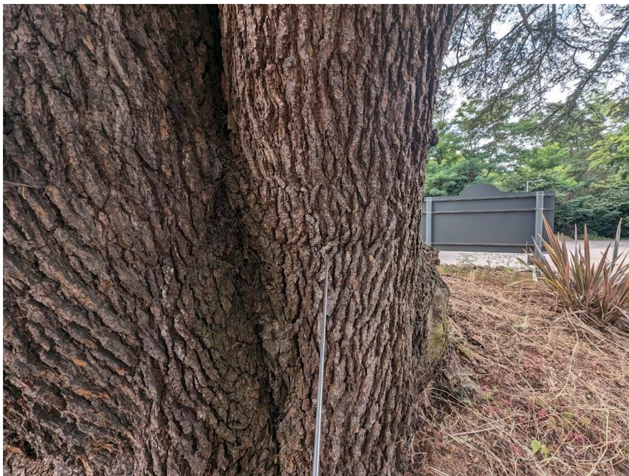
Figure 11: Fibre buckling, 12.1 in findings
