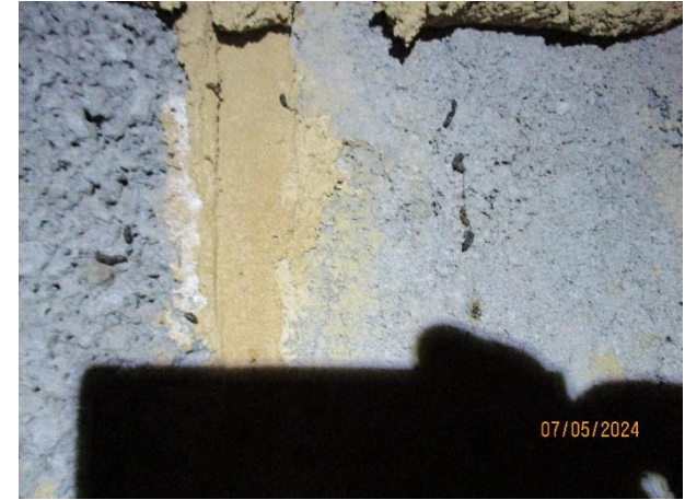
Photo 21: Bat droppings within Main Void.
