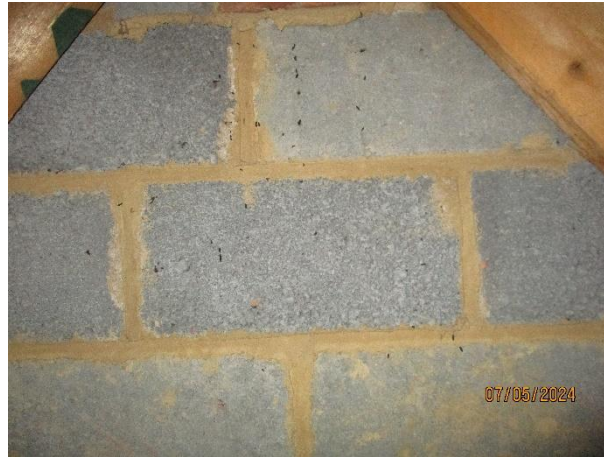
Photo 20: Bat droppings within Main Void.
