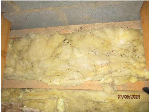
Photo 19: Bat droppings within Main Void.
