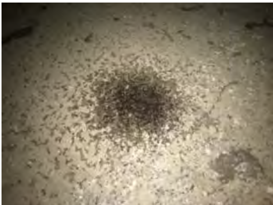
Photo 72 Building B3 – clustered bat droppings
