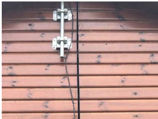
Photo 83 Building B8 – split in panelling
