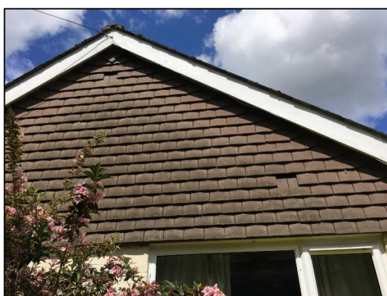
Photo 37 Slipped tiles (B1)
