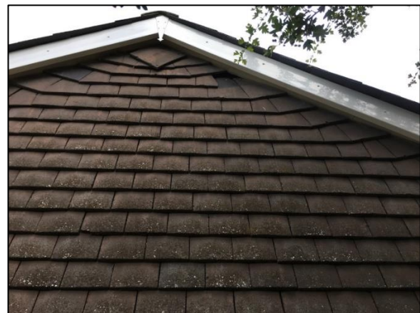
Photo 66 Bird nesting behind slipped tile
