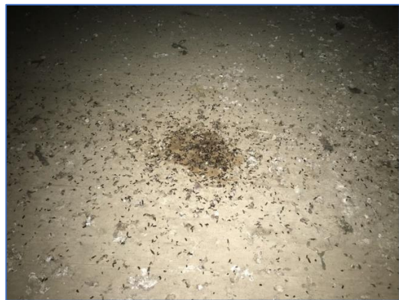
Photo 54 Cluster of bat droppings pile 2 (B3)
