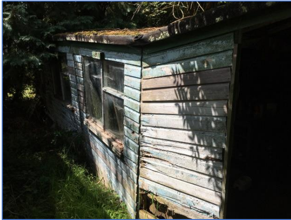
Photo 57 Dilapidated structure (B5)
