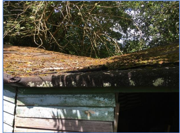
Photo 58 Dilapidated structure (B5)
