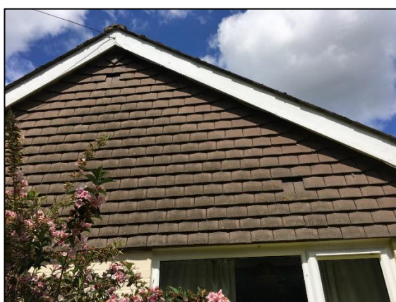
Photo 37 Slipped tiles (B1)
