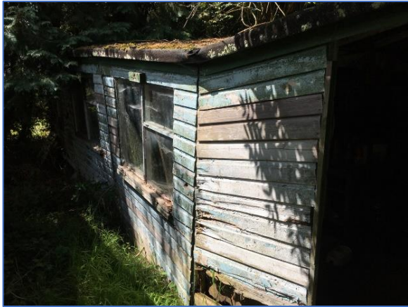
Photo 57 Dilapidated structure (B5)
