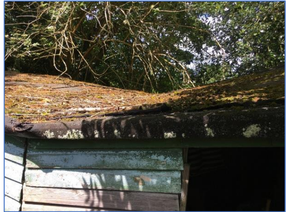
Photo 58 Dilapidated structure (B5)
