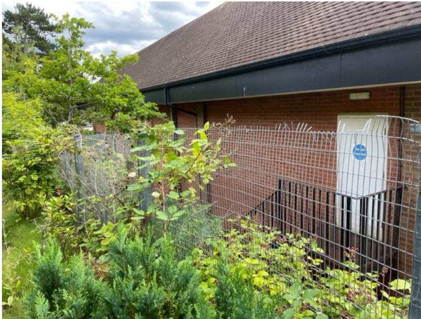
Figure 1 showing existing 1st flr fire escape door with existing ground floor one directly below facing into a steep bank
