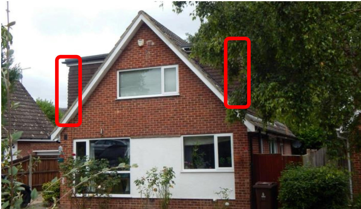
Image 3 – North facing elevation of the property offering further gaps within the vertical hanging tiles
