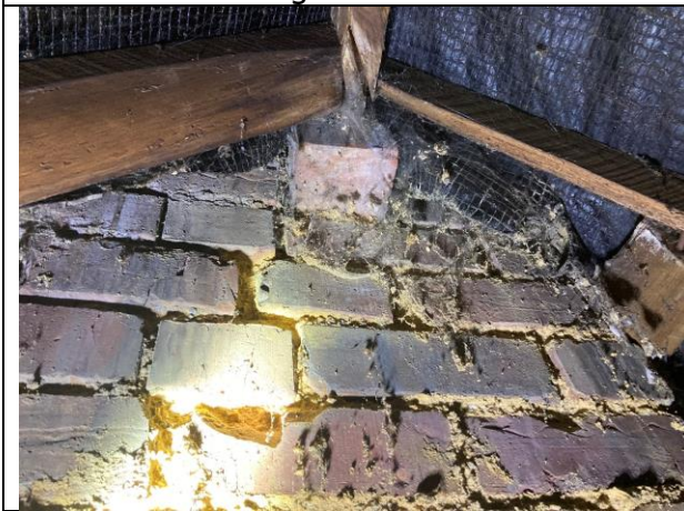
Photo 5 Cobwebs across gaps
