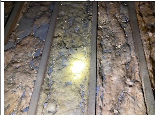
Photo 7 Old dust at loft floor
